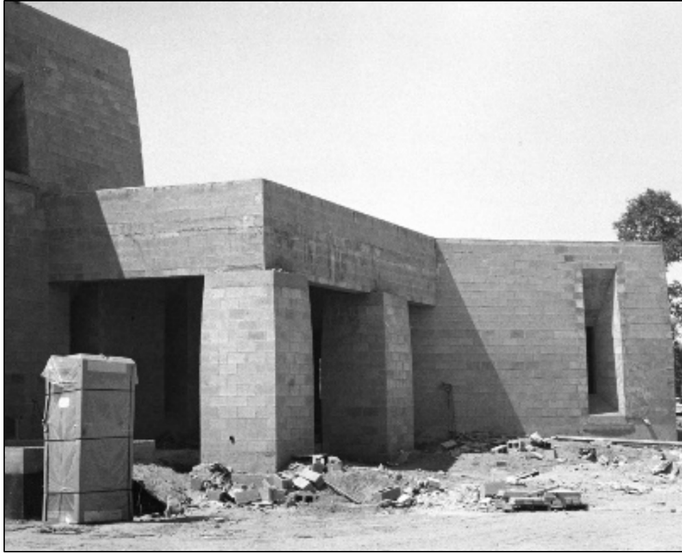
Photo 31. View of the north elevation under construction with the porch opening c. 1968 (Scottsdale Public Library)
