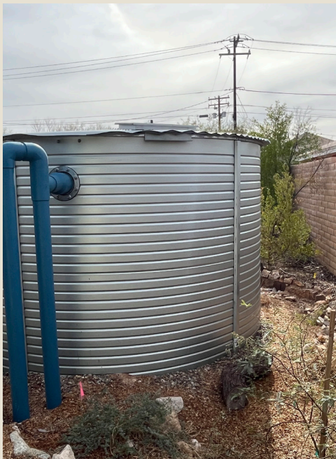
Above ground cistern.
