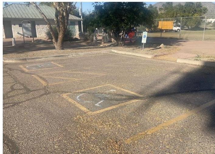
Fading Accessible Parking Spot Paint
