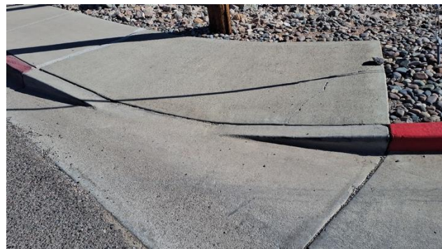
Curb Ramp with Missing DWS
