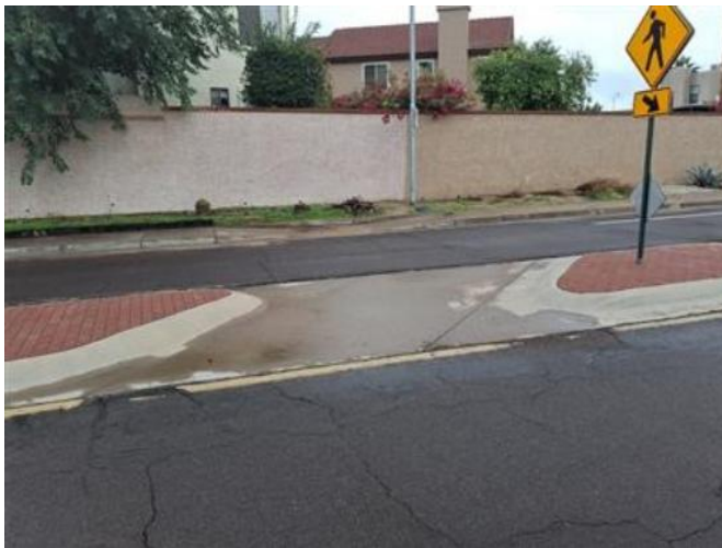
Median Refuge Island with Missing DWS
