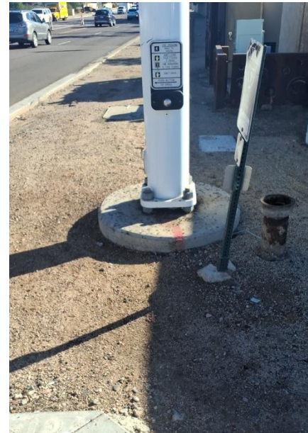
Push Button with no pedestrian access
