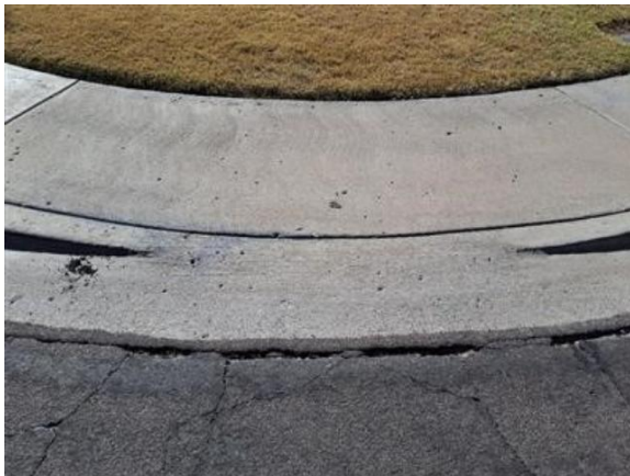
Diagonal Curb Ramp with Missing DWS
