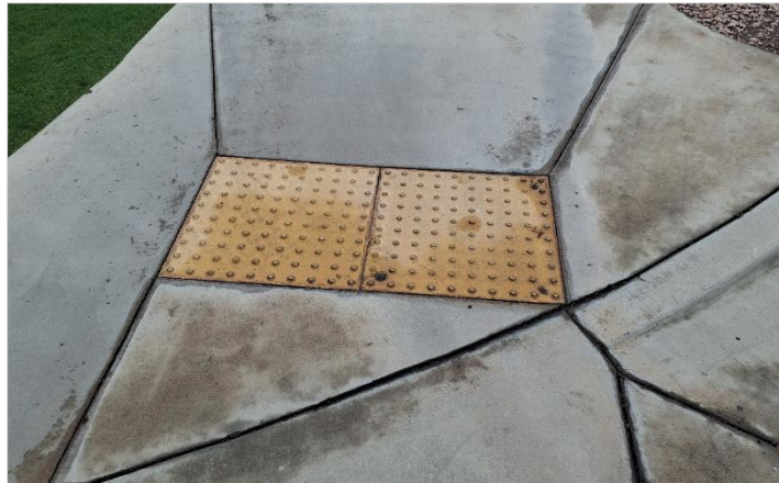
Perpendicular/Directional Curb Ramp with a 17.6% Running Slope
