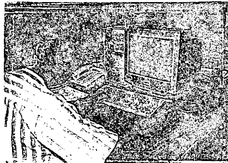
One of many terminals of the Supervisory Control and Data Acquisition System (SCADA) used to control the entire water production, distribution and wastewater collection system.
