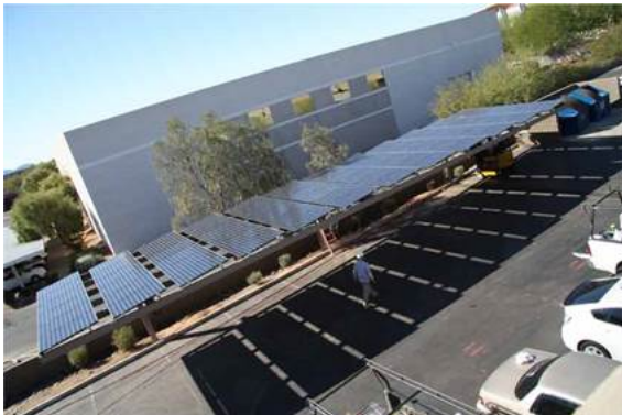
Solar PV carport structure.
