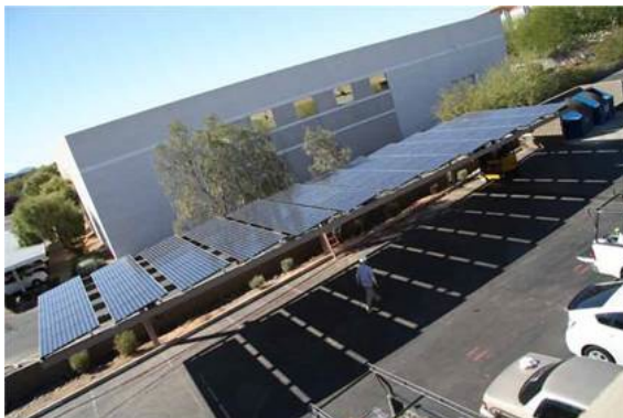
Solar PV carport structure.
