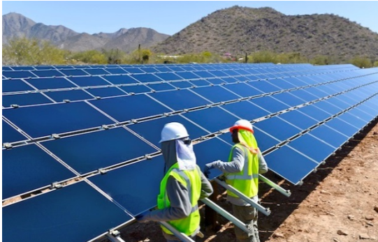
Ground mounted solar PV system.
