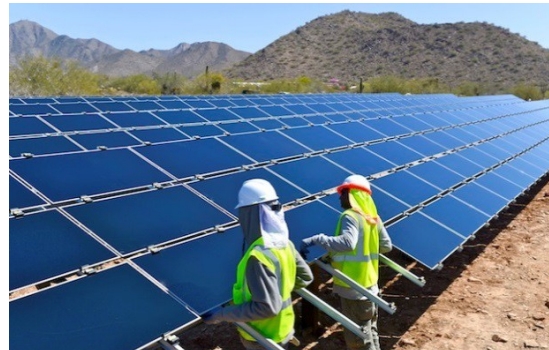
Ground mounted solar PV system.
