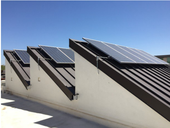
Roof top building integrated system.
