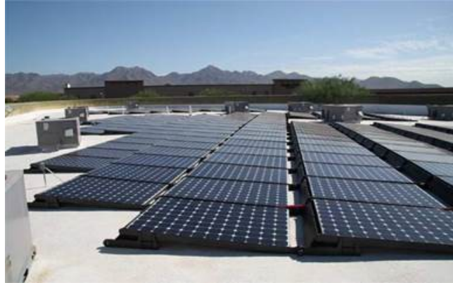
Solar PV rooftop installation below roof parapet.
