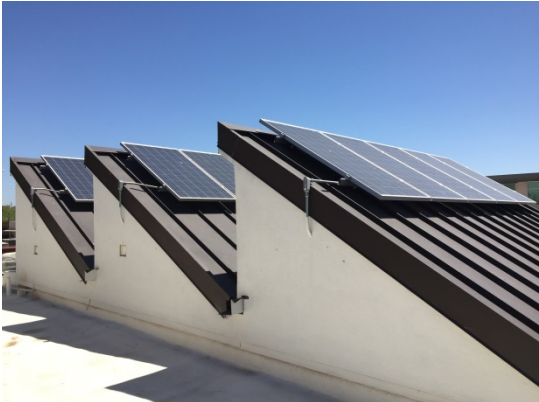
Uniform solar panels aligned with roof slope.
