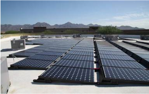
Low-slope solar PV panels below roof parapet.
