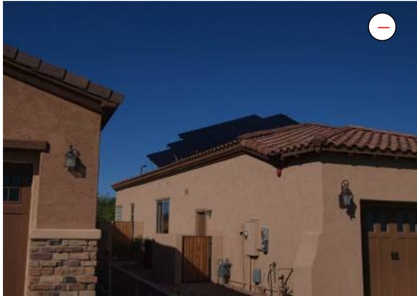
View from southwest corner Solar panels on west facing pitched roof exceed the maximum allowable height of 24 inches above roof surface at any point.
