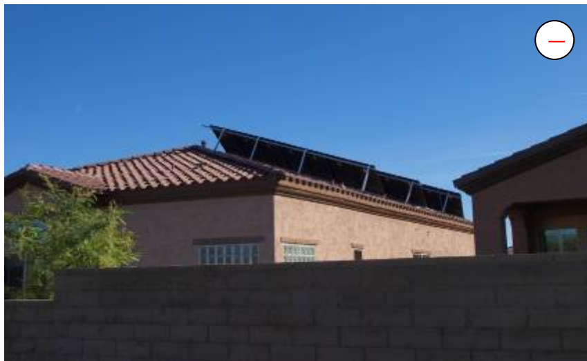
View from northwest corner Solar panels on west facing pitched roof also project above the roof ridge line. Support structure color is not compatible with roof surface color.
