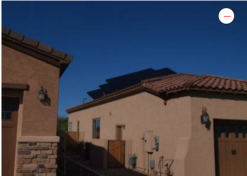
View from southwest corner Solar panels on west facing pitched roof exceed the maximum allowable height of 24 inches above roof surface at any point.
