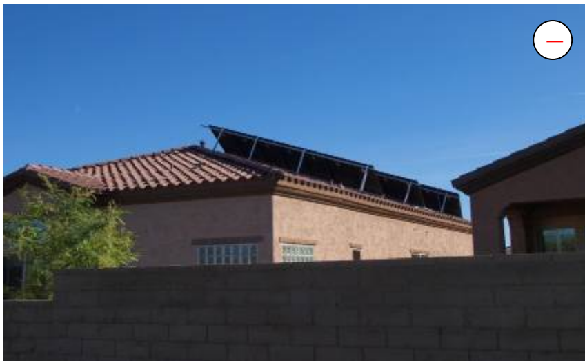
View from northwest corner Solar panels on west facing pitched roof also project above the roof ridge line. Support structure color is not compatible with roof surface color.
