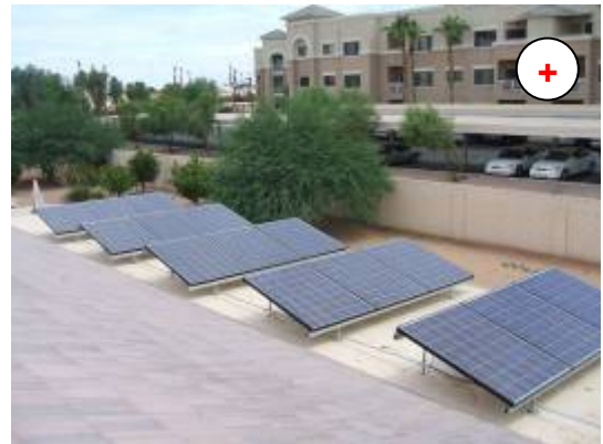
Solar panels on flat roof without parapets.
