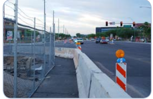
Capital improvements, such as roadway construction and pipe upgrades, should be coordinated whenever possible.
