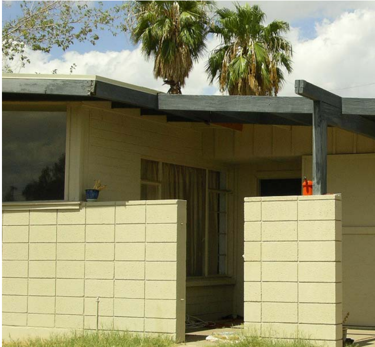
This entry is in original form, including the exposed rafter that was intended to be both ornamental and structural.
