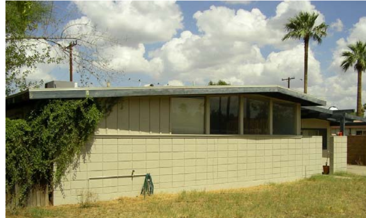
One of the most intact of the Town and Country residences, this house features simple but Attractive concrete block at the base, board and batten on the upper wall, the original window band and the original open entrance.
