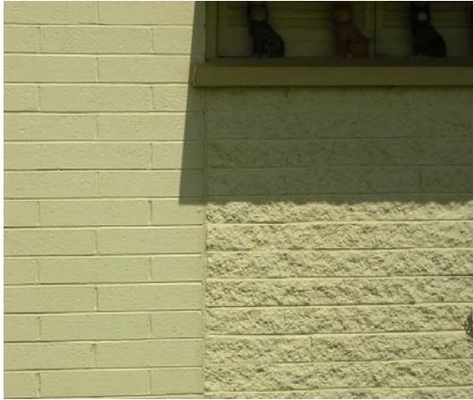
Mismatched block texture should be avoided
