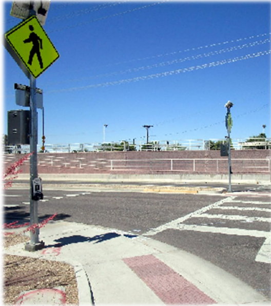
Rectangular Rapid Flashing Beacon
