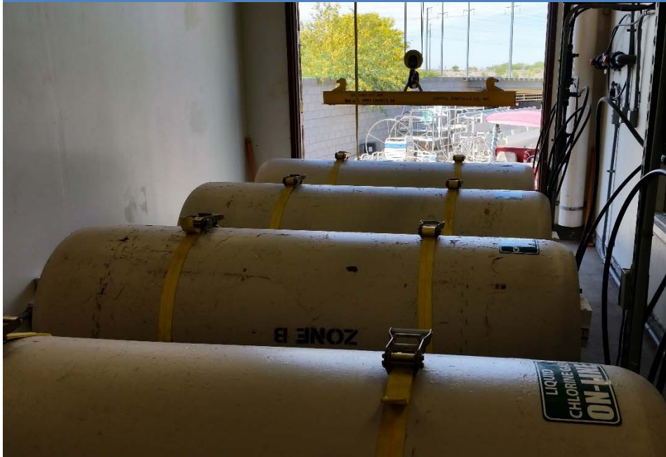
Above: Old gaseous chlorine tanks
