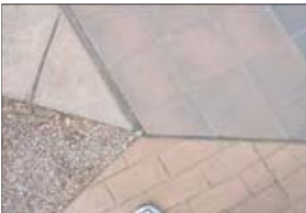
Avoid placing multiple paving surfaces in the walkway.
