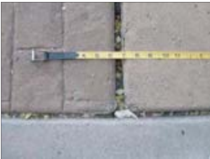
Avoid overly textured sidewalks with cracks or indents greater than 1/4".
