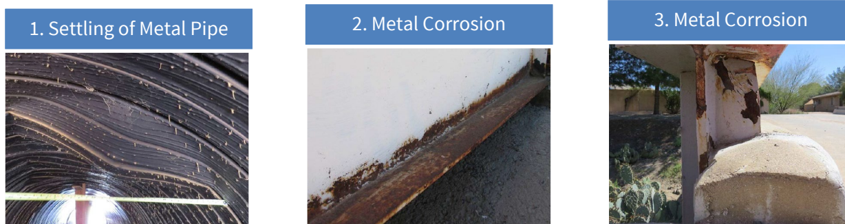
Figure 8. ADOT Bridge Inspections with “Structurally Deficient” Classifications
