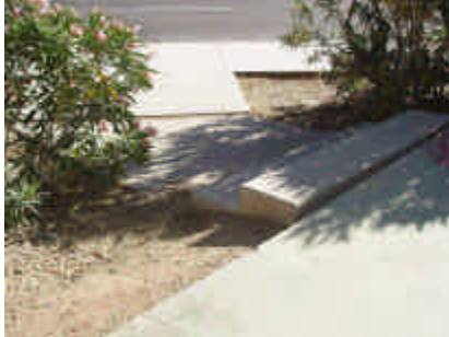
Northeast Quadrant – unsafe pavement joint
