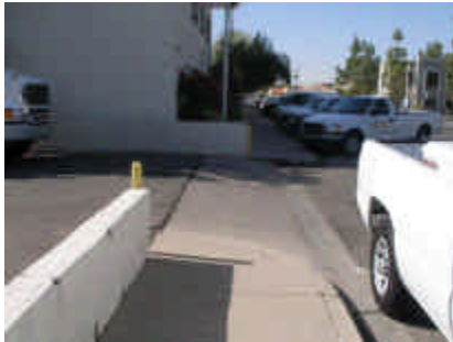
Northeast Quadrant – lack of ramps
