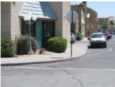
Northeast Quadrant – lack of ramp
