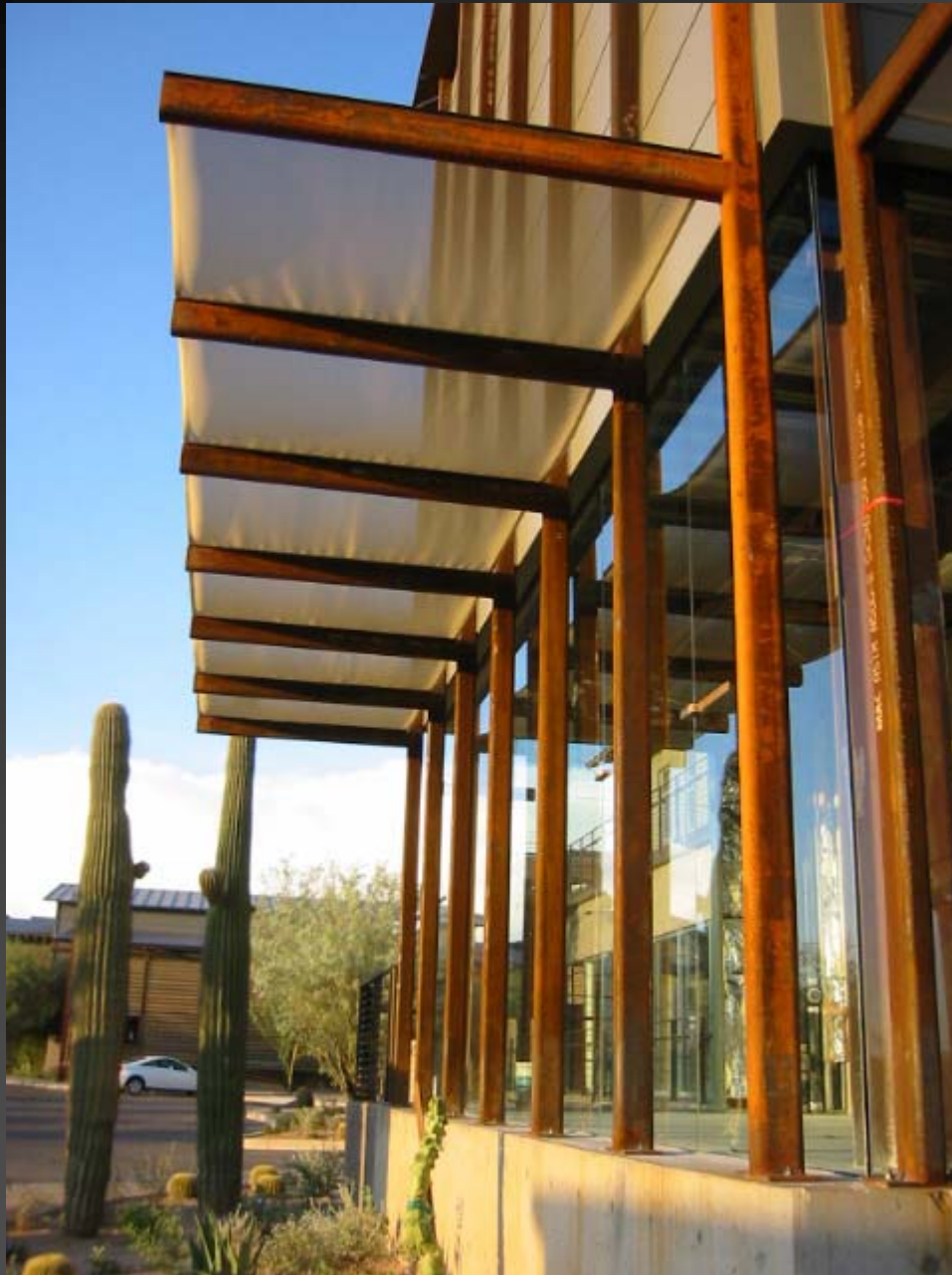
Insufficient Shading on West Elevation at DC Ranch
