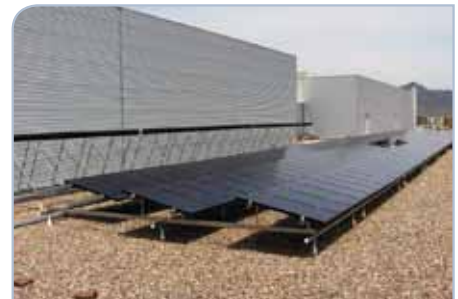
Alternative energy generation, such as solar power, can help reduce peak electricity demand and save on energy costs. Photo source: Henkel.
