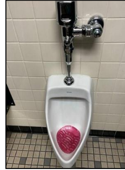
Flush Valve Urinal
